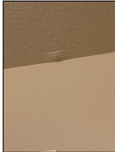
Nail pops noted at upper level ceiling area.
