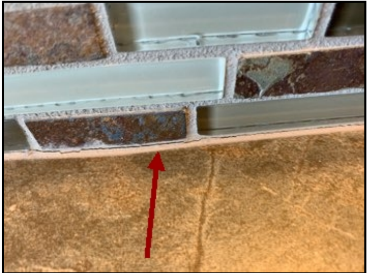
Caulk or grout at/or behind sinks and master tub as needed.
