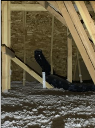
Properly vented to exterior of structure.
