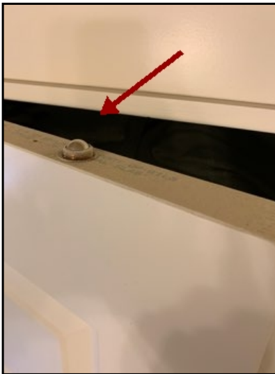
Door hardware needs adjusted at upstairs hall closet door.
