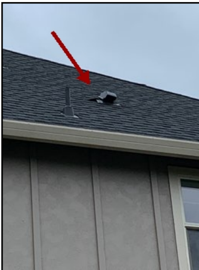
Roof vent on left side of structure appears loose and pulling away. Recommend repair.
