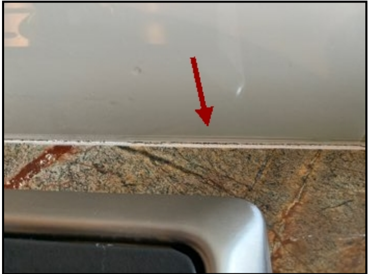
Caulk/Grout is needed at kitchen backsplash. Caulk as needed.
