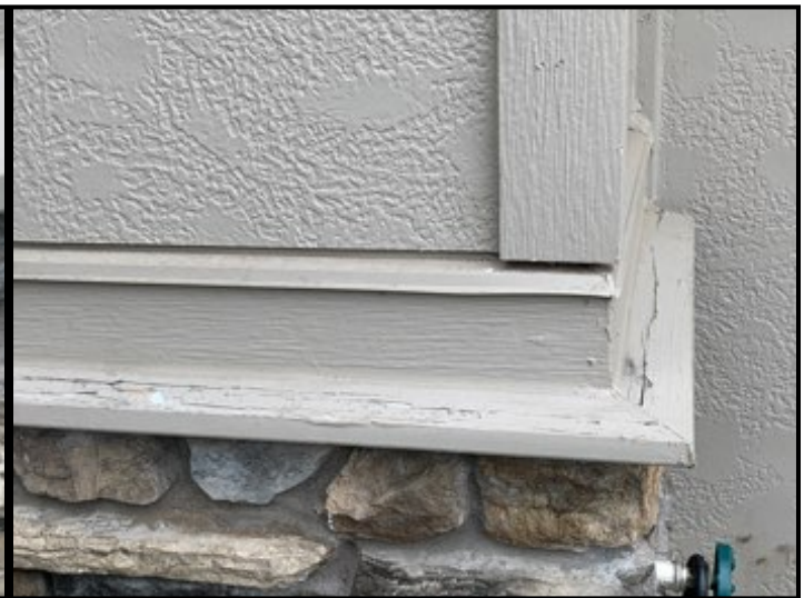
Peeling paint observed on trim. suggest scraping and painting as necessary.
