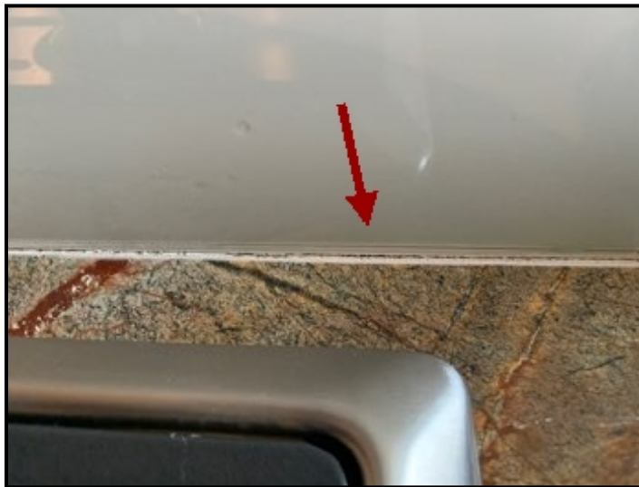
Caulk/Grout is needed at kitchen backsplash. Caulk as needed.
