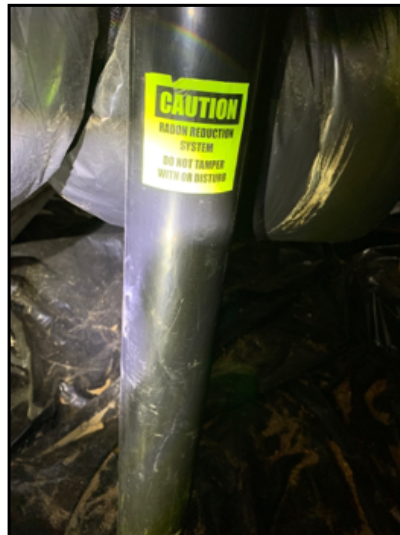
Passive radon vent noted.
