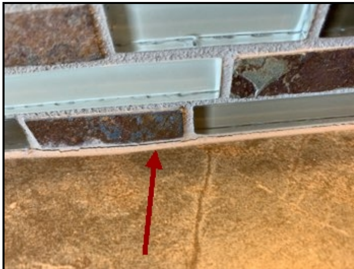
Caulk or grout at/or behind sinks and master tub as needed.
